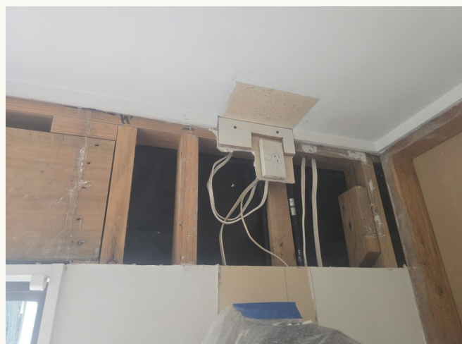
Wall opening and services exposed | Forrest Hill
