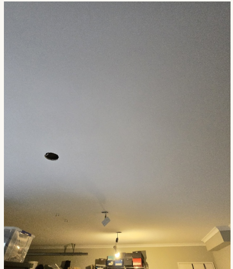
Later painted ceiling surface
